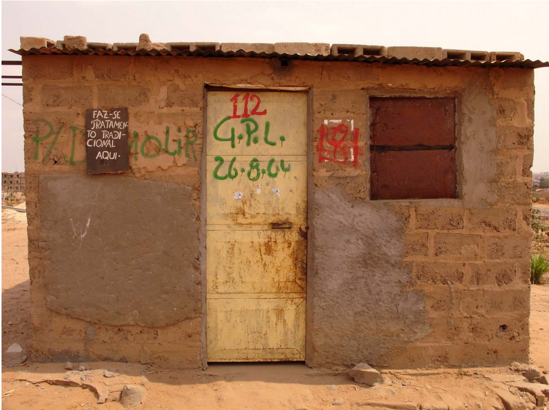
House marked for demolition by the Provincial Government in Mbondo Chape. © 2006 Paula Martins/Human Rights Watch
